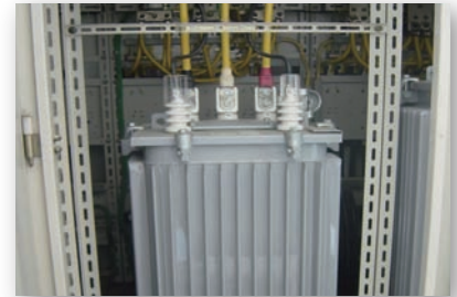
High efficiency transformer at the Mie plant
